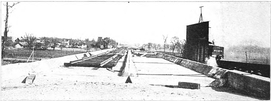
Fig. 29—Concrete Slabs on Deck Plate Girders for Ballasted Floor, C., M. & St. P. Ry.
