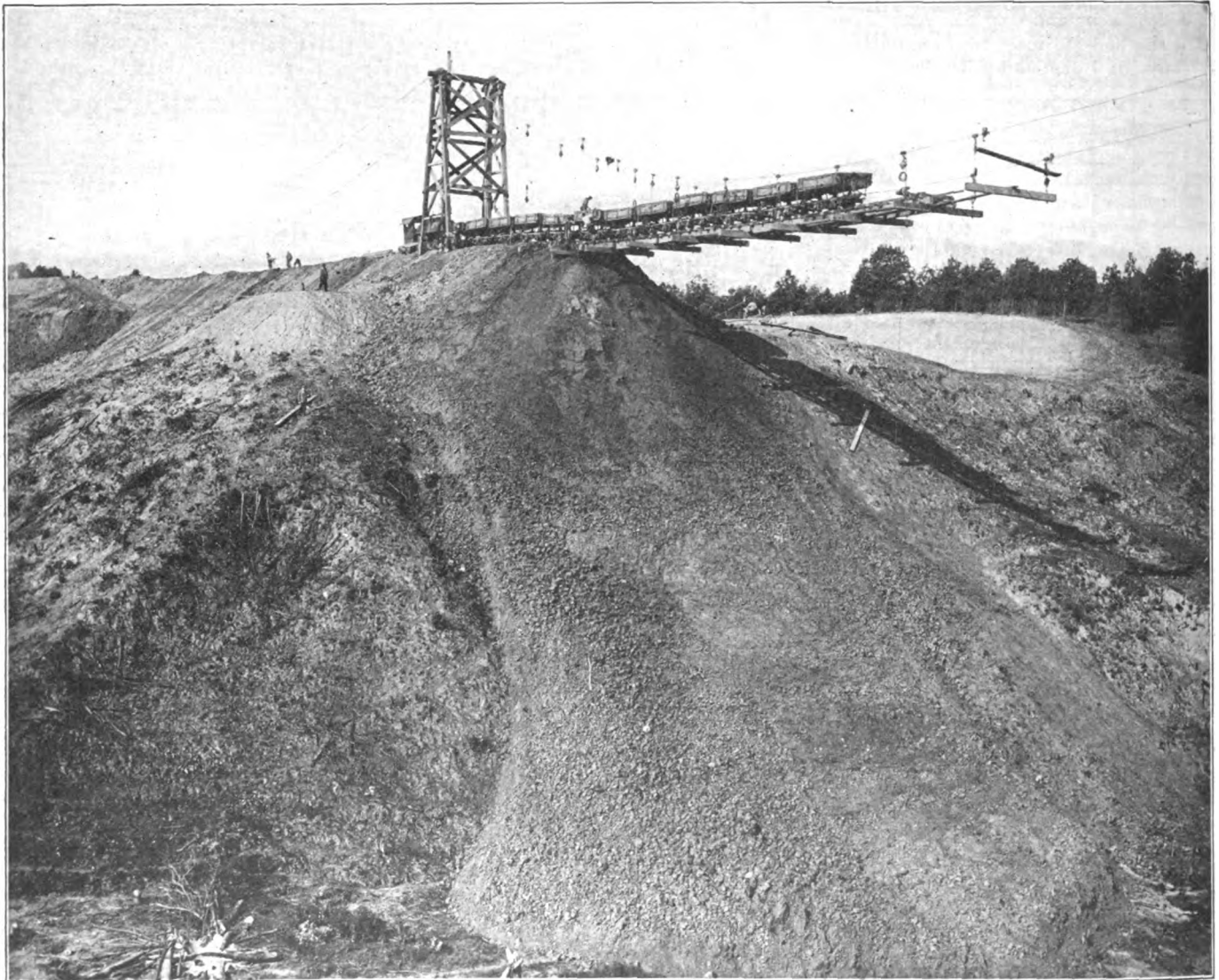
Dumping Cable Making the West Approach Fill to Des Moines River Bridge
