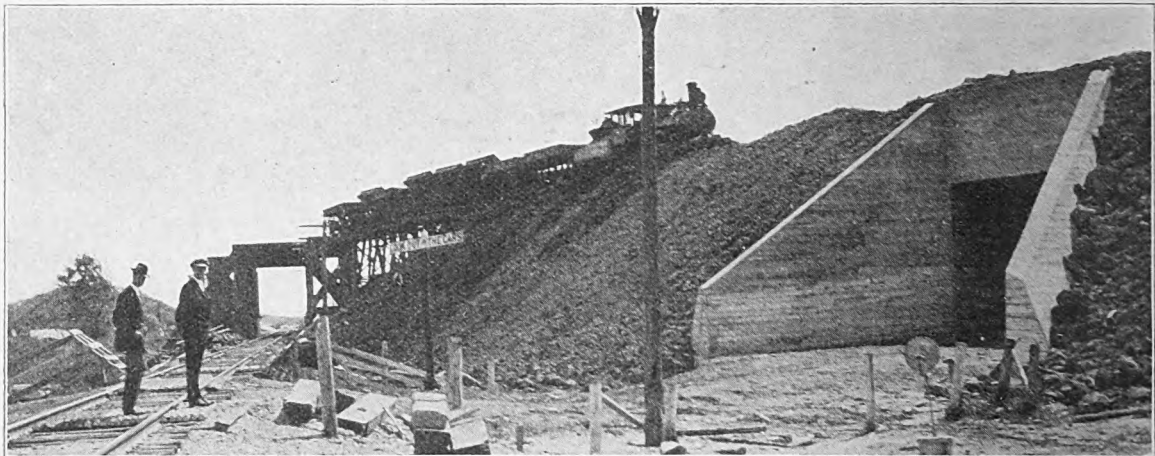
Fig. 7—Highway Under Crossing (In Foreground) and Overhead Crossing of Operated Line Beyond.
