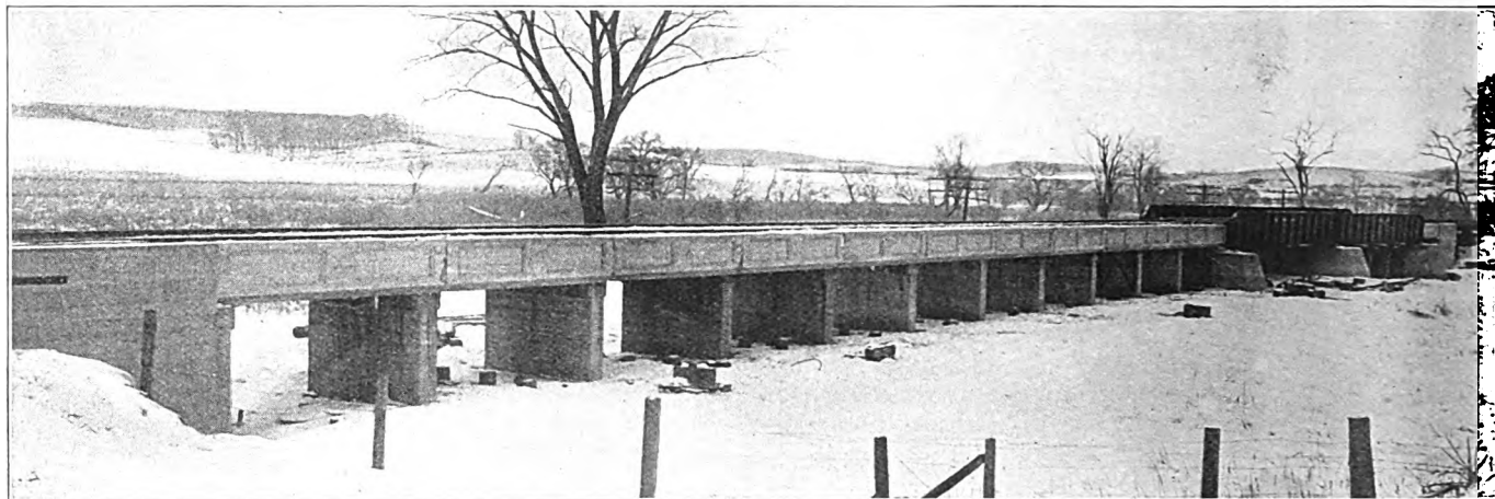
Fig. 32—Type of Concrete Trestle, with Ballasted Deck, C., M. & St. P. Ry.
