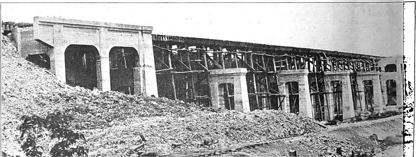
Fig. 35—Skunk River Bridge, Near Cambridge; Progress View; Five 75-Foot Deck Plate Girders, with Concrete Slab Deck
