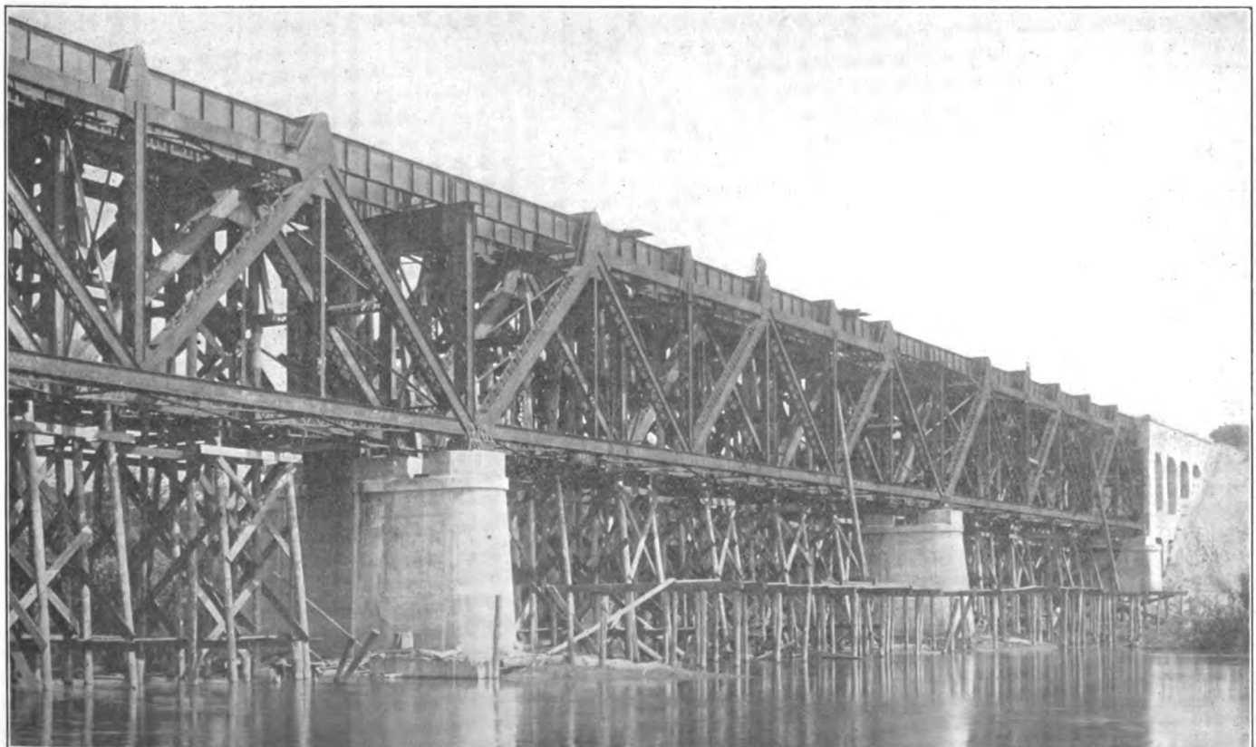
Part of the Cedar River Bridge Showing Timber Bents Supporting Floor Beams During the Construction Work and Concrete Blocks on Piers used to Raise the Elevation
